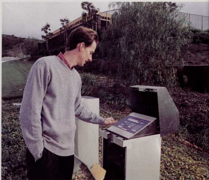
Irrigation consultant Steve Hohl programs one of over 300 Rainmaster Evolution controllers being installed for the Ladera Ranch project.
