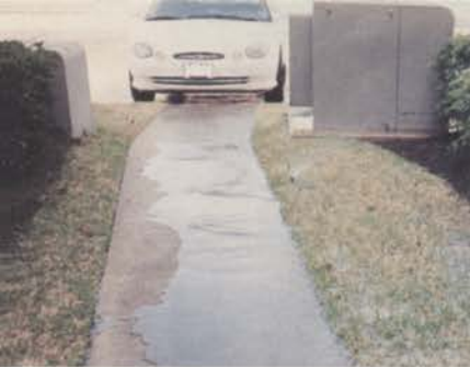
This flooding was caused by a broken underground pipe. It was detected during the site inspection phase of the irrigation audit.
