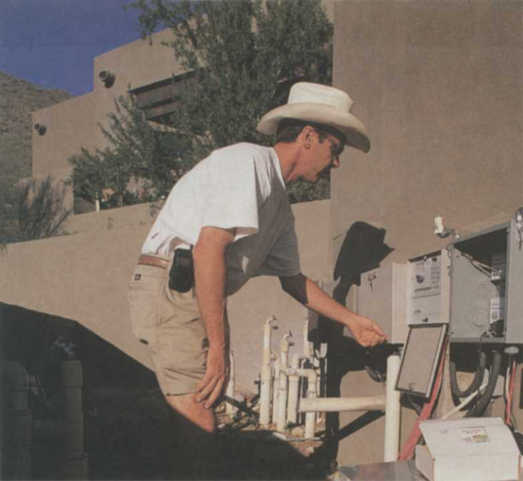
Dickey adjusts drip schedule at the controller, where many drip inefficiencies originate.
