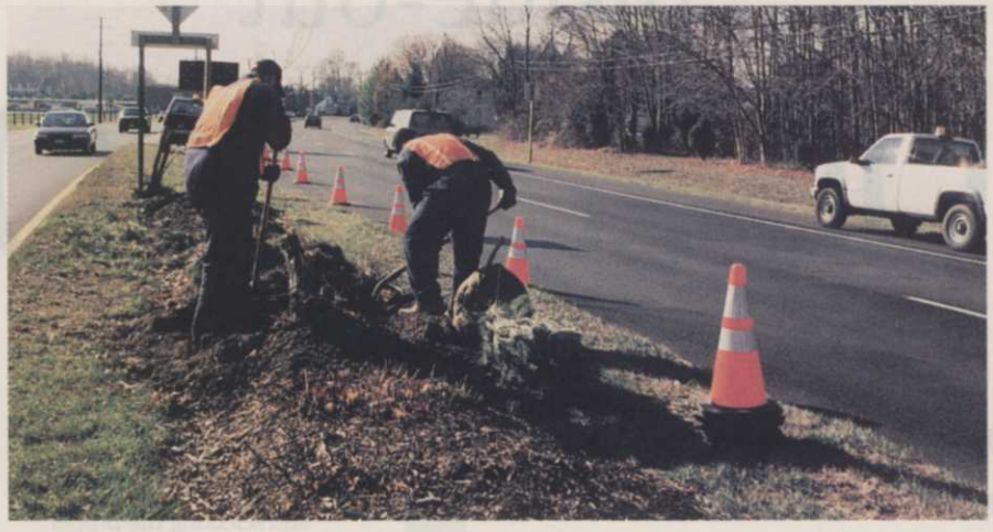
Stan Speaks and Ronald Offer of Anne Arundel Co. Central Services work on Solomon's Island roadway median, where signage and visibility are important for safety.
