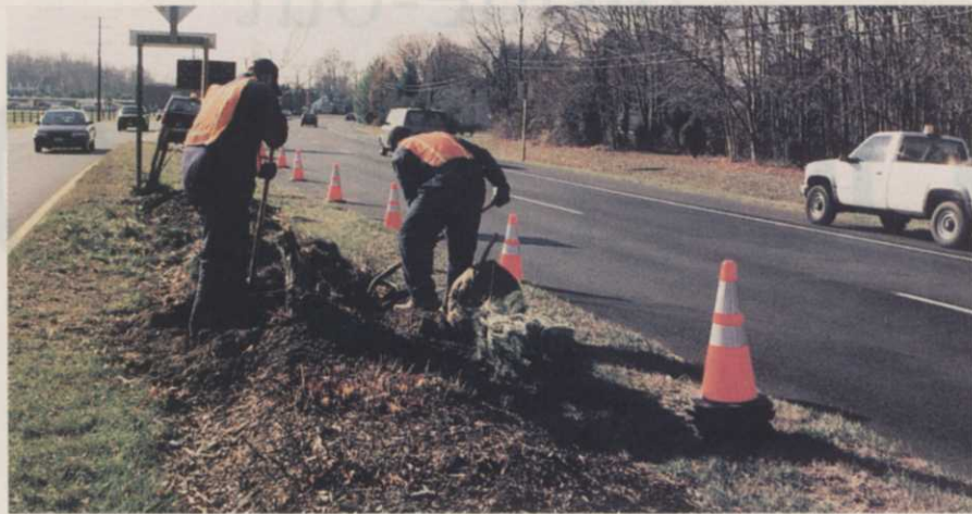
Stan Speaks and Ronald Offer of Anne Arundel Co. Central Services work on Solomon's Island roadway median, where signage and visibility are important for safety.
