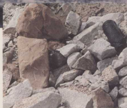
Debris like this is becoming an increasingly common problem at job sites.
