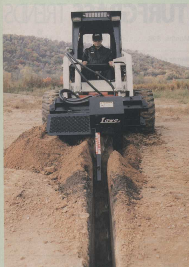
The Lowe Model 7 hydraulic trencher adds versatility to smaller skid steer loaders in the 800- to 1000-lb. class.
