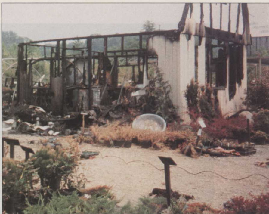
This damage, and that on page 15, was not caused by an accident. It was deliberate, an act of vandalism. It occurred in a nursery/landscape company in the East several years ago.
