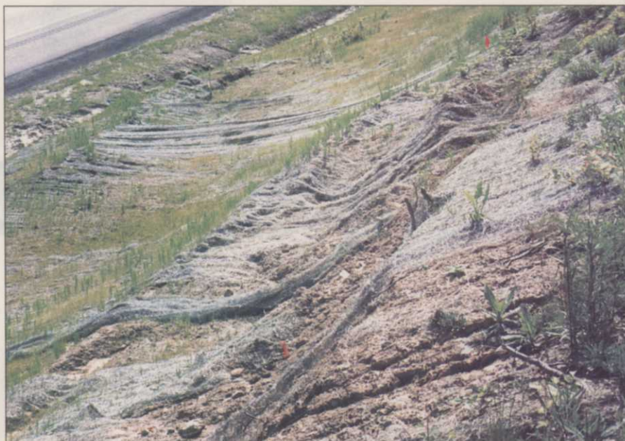
Correct installation of materials is essential for successful control of soil erosion. Heavy spring rains devastated this newly planted roadside even though a fabric covered it.
