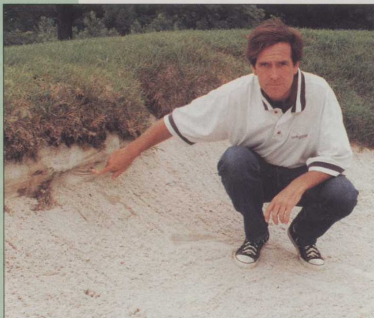
Kelch shows the filter fabric liner at hole 17 that has become exposed due to raking. It's tough to keep the grass wet and growing over the liner, says Kelch. The liners will be removed before the Bell Atlantic tourney.
