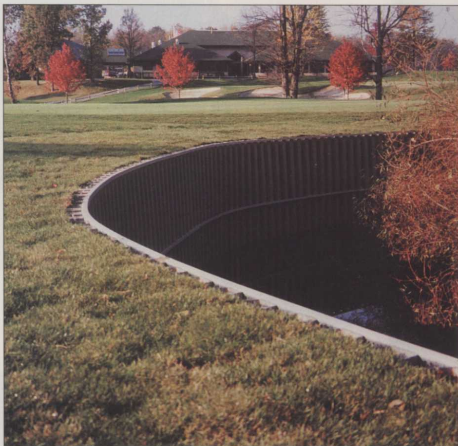
After the fill had settled, it was topped with soil and sodded.
