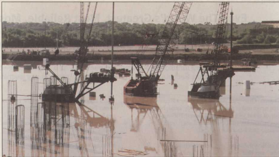
The Miller Park construction site filled up with 10 feet of water. It helped save the Brewers field from further flooding.
