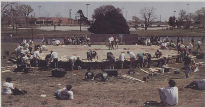
Student Career Days contestants competed in 20 events, including a wood construction competition on an outdoor stage.
