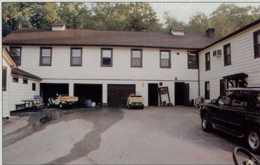
The original building was remodeled to be used as an administrative building. That project included a new roof, new gutters, vinyl siding, new windows and interior work.
