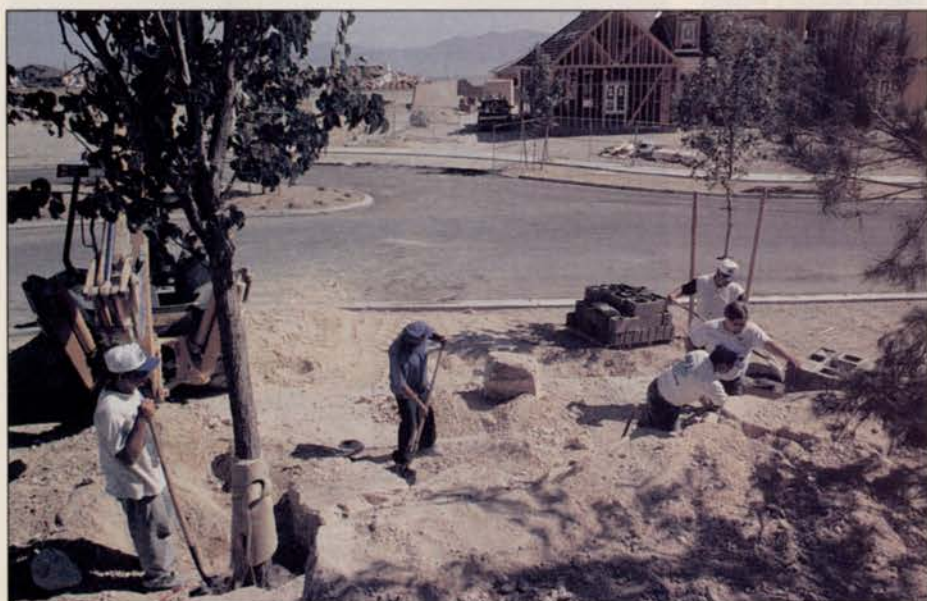
A Par-3 Landscape residential construction site in the Mountain Trails subdivision—workers installing mature trees to give a finished look to an upscale job
