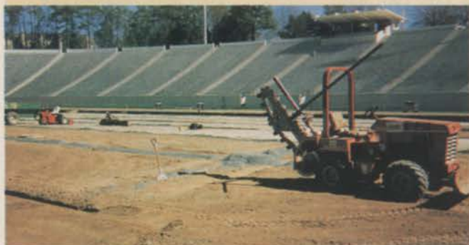
"Everything on the Duke field drainage project was local," says contractor Nolan Thomas. That includes the pipe, rocks, sand and crew.
