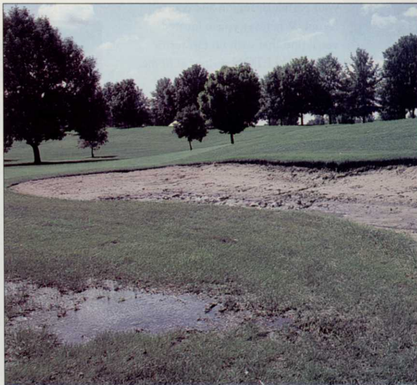
Wet bunkers that drain poorly are tough to maintain and are a constant source of golfer complaints.
