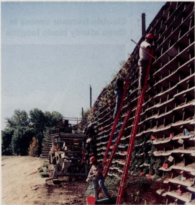
Kuehne Company built this 22-foot-high traffic noise barrier using triangular-shaped frames of recycled plastic called Recy-walls by Sanders Enterprises Inc.
