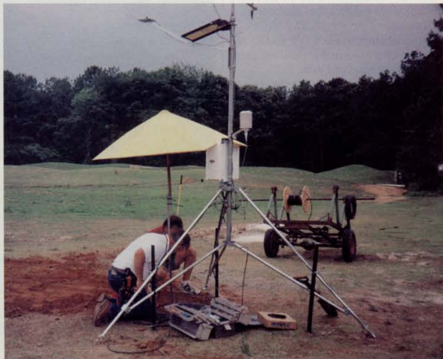
Workers install the Georgia Turfgrass Foundation Trust's new weather station adjacent to its research green in Duluth. Photo by Doug Moody
