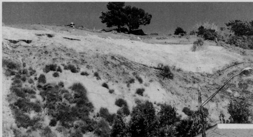
Poz-O-Cap, in the white area, was applied to a half-acre hillside in Malibu to prevent soil erosion.
