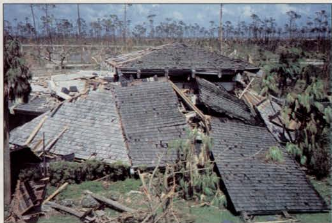
Hurricane Andrew destroyed the zoo's Lakeside Restaurant.
