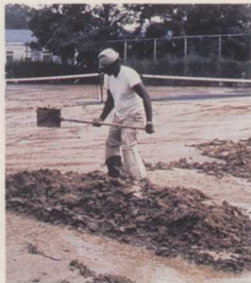
Soil erosion ruined this tennis court.
