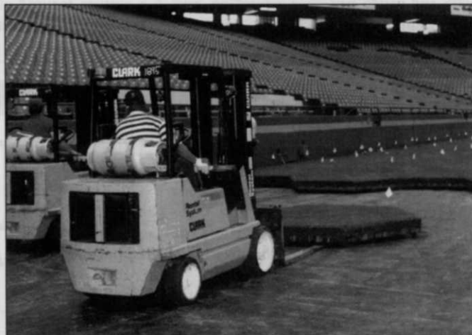
A fleet of forklifts positioned each of 2,000 separate pieces of sod into a rectangular carpet of turfgrass.
