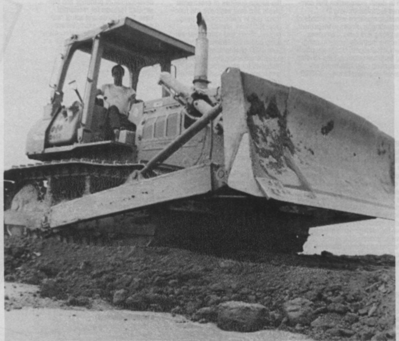
About six inches of backfill was bladed onto the geotextile, spread in the direction of its overlap to keep the fabric from separating.
