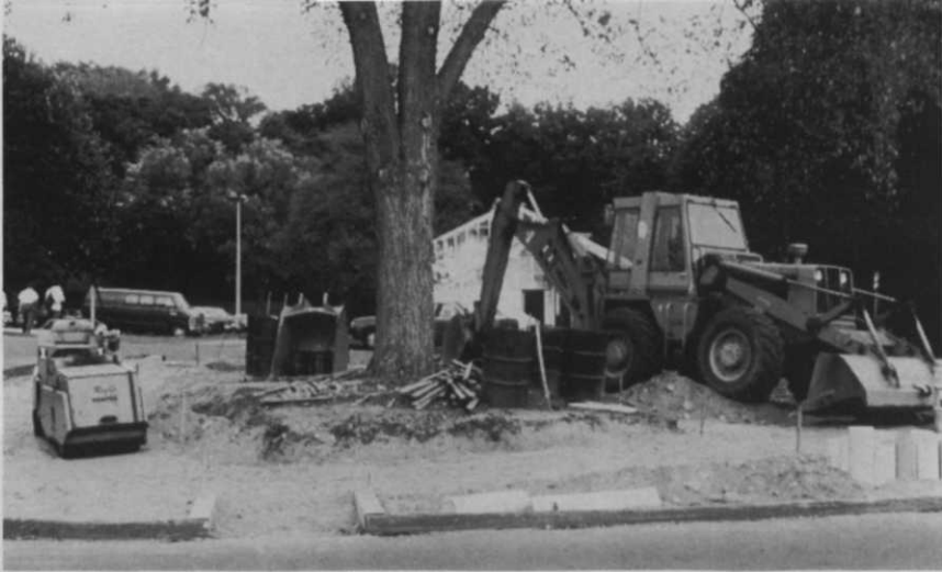
Construction remains one of the biggest threats to trees. Injuries are caused by raising or lowering of grade and by trenching near the tree. Still, injured trees may take years to die.
