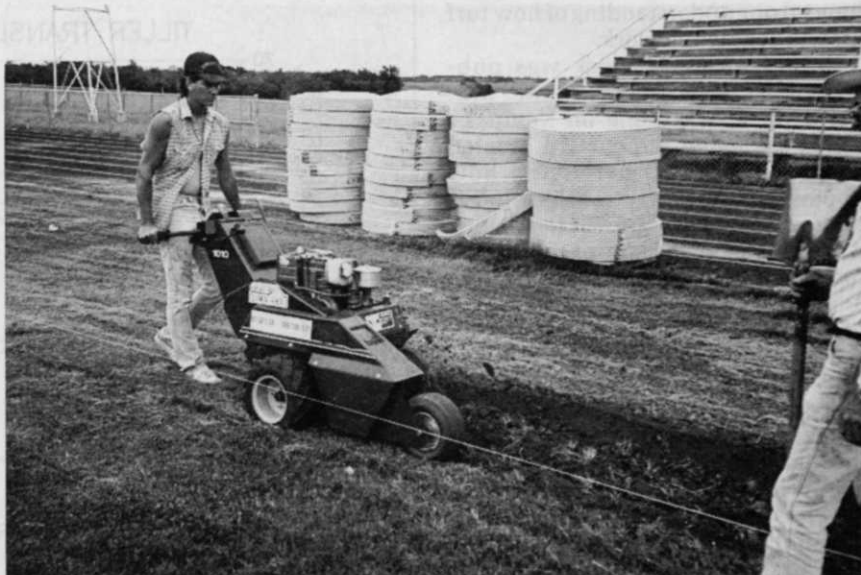
Digging the trench for the 12-inch TerraFlow trunk line along one sideline using the Ditch Witch 1010 trencher.
