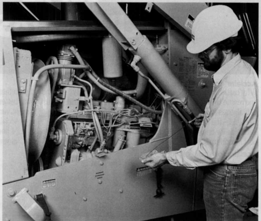
Unexpectedly low oil levels are a sign that a leak needs attention. Excessive oil use or very dirty oil is a cause for concern.
