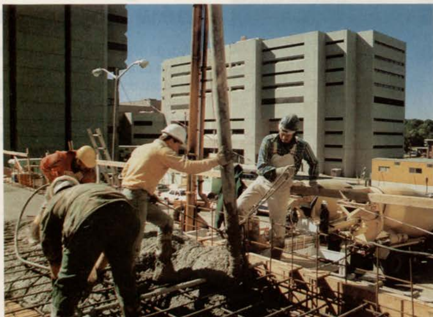
Concrete is poured with the use of a concrete pump tank (in background). Notice two concrete trucks pouring at the same time.
