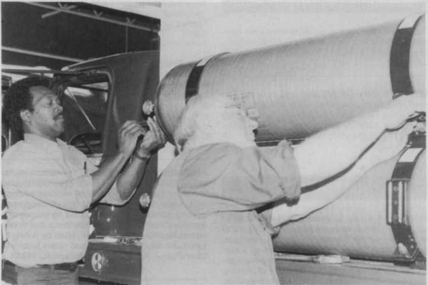
Tanks for storing natural gas are installed as a part of the conversion to dual fuel operation by participants in a seminar on natural gas conversion at Hocking Technical College in Nelsonville, Ohio.
