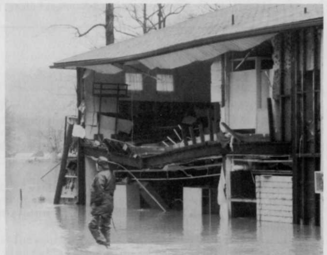
A worker surveys damage to the clubhouse where water reached the second floor.
