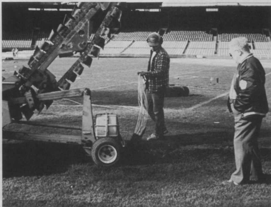
Harry Gill (right) supervises installation of the irrigation pipe and wires through slit sod. "The only places we had to remove the sod was when we came to a sprinkler head," Gill notes.
