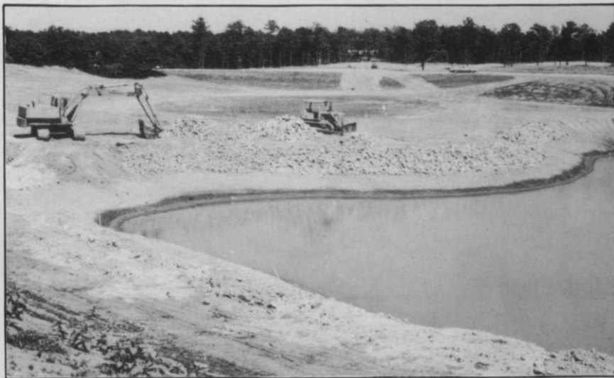
Surface water at Dennis Highlands is piped into a retention pond in a low area of the course for future irrigation purposes. The pond also reduces wind evaporation of the water and adds to the surrounding scenery.
