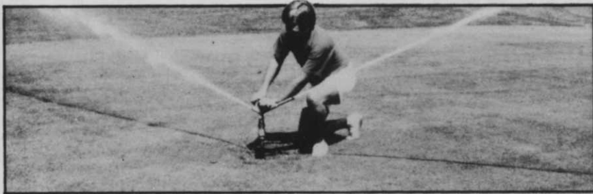
Pakkala locks in head to manual irrigation system. An automatic system is part of the reconstruction plan.
