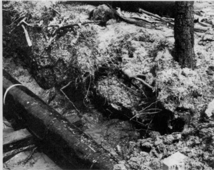
Underground utilities often cut many tree roots and cause a decline in nearby trees.
