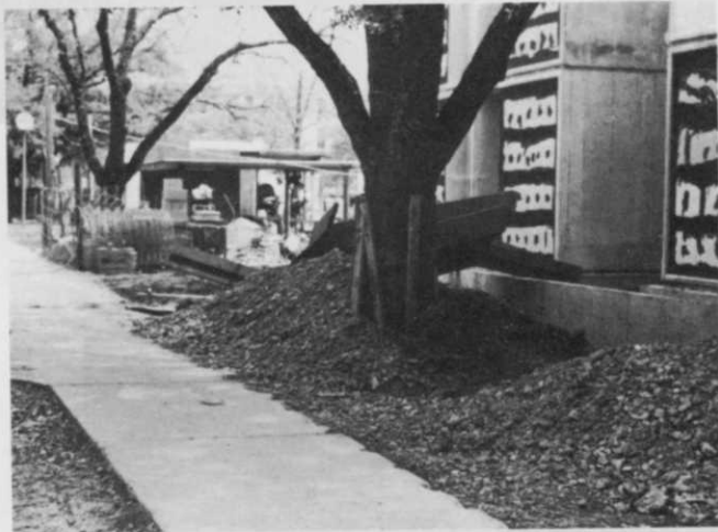
Trunk protection cannot offset the root damage caused by sidewalk and foundation construction. Dieback is already evident before construction is completed.
