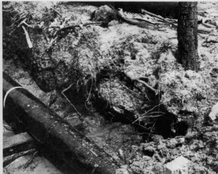
Underground utilities often cut many tree roots and cause a decline in nearby trees.
