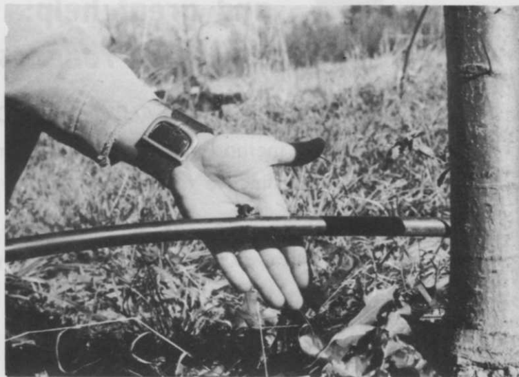
Emitter , inserted directly into laterals through a hole punched at the base of each tree, simplifies and shortens the installation process.
