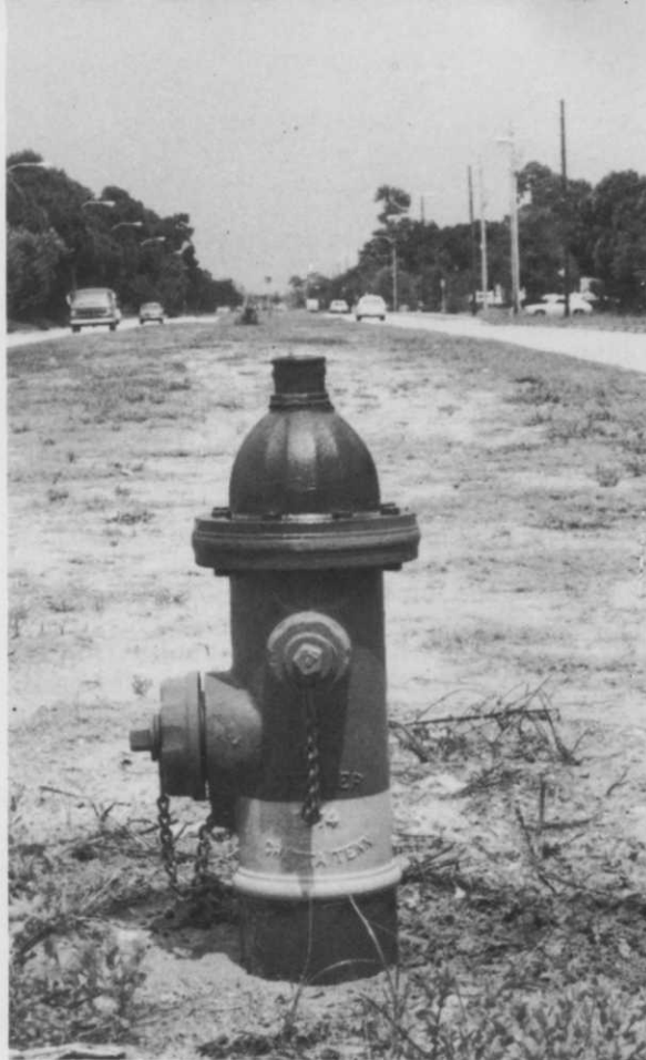
One of the many outlets to the 14-mile distribution system for the recycled wastewater.
