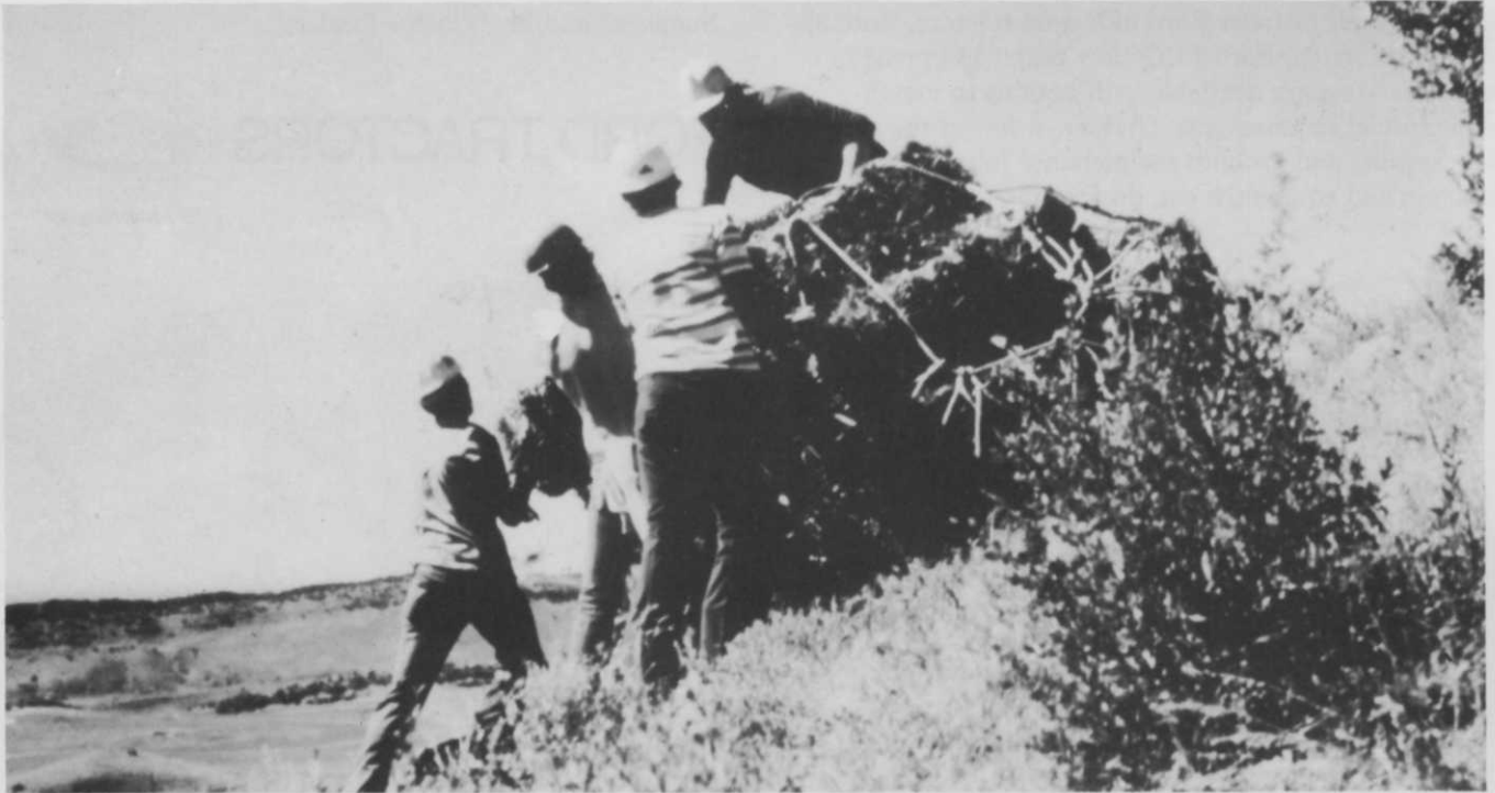
Workmen on hillside unload materials brought to the site by helicopter. Use of the helicopter preserved the slope from additional wear.
