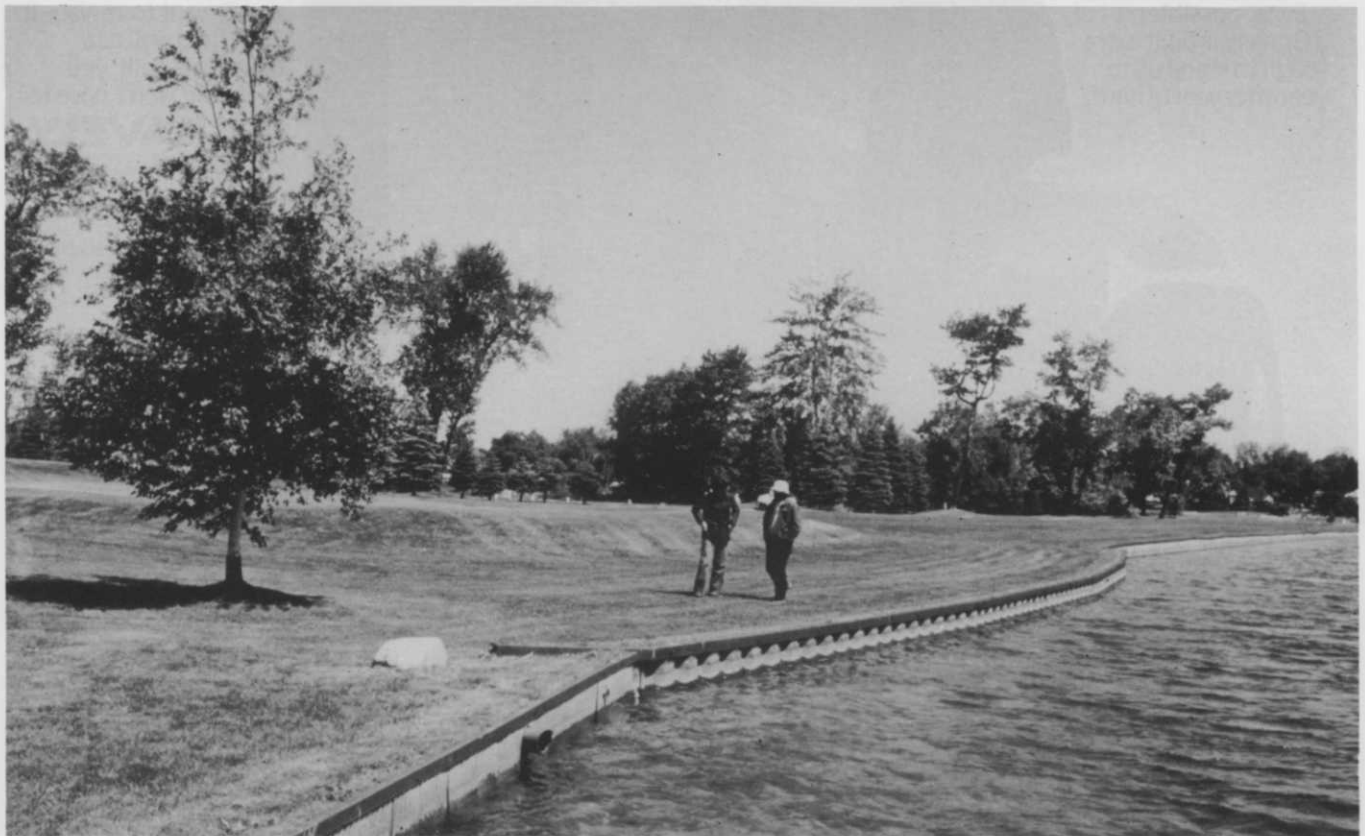
Corrugated sheets (lower left) show more wear even though they were installed after the piling (center).
