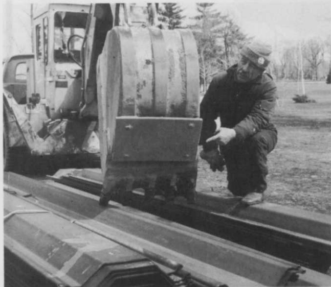
Bay Pointe superintendent Don La Fond Explains use of heavy steel plate on backhoe bucket to drive piling around ponds.
