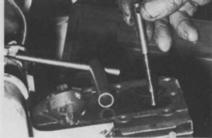
It is also necessary to reface the valve seat. The tool shown is inserted in three pieces. First the pilot.
