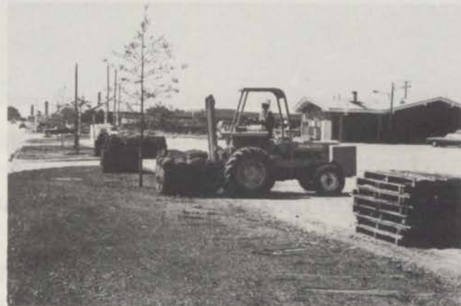
Forklift picks up a fresh pallet of sod to carry 200 yards up the road to installers.
