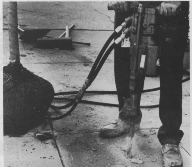
After the sidewalk has been scored and cut, the jackhammer is used to break-up the concrete.
