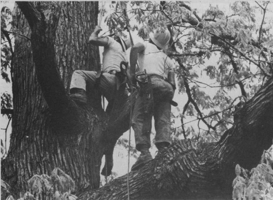
Lightning protection installation comes naturally. It fits the knowledge, tools, skill and experience of tree climbers.
