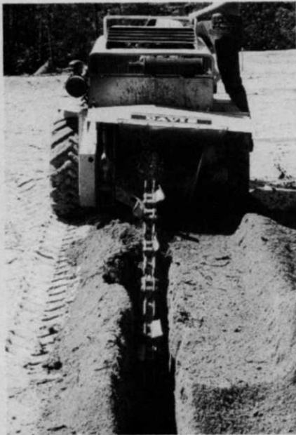
A trenching machine was the only piece of special equipment required to lay the irrigation system's pipe network.
