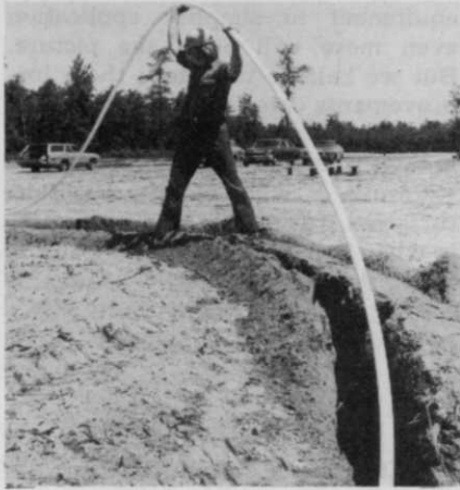
The flexibility of PPC means the pipe could easily bend around greens on King's Grant Golf Course.
