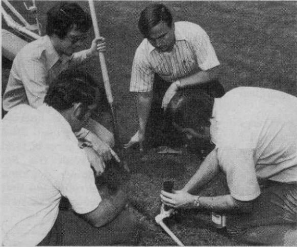
Students actually install an irrigation system as part of their training. Practical experience such as this is invaluable in understanding the problems installers have.
