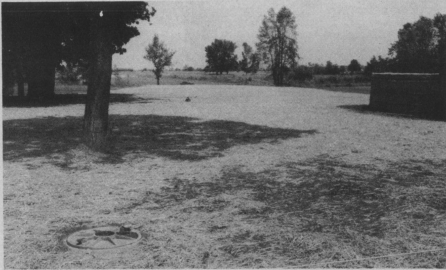
This area was seded and covered with straw following placement of the sewer project. Contractors followed stander seeding specifications to restore site to the original state.
