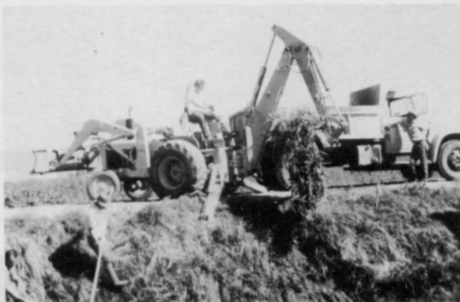
Work crews from the Lower Tule Irrigation District remove alligatorweed with a backhoe. Mats of the weed become so thick that water cannot flow along the ditches.
