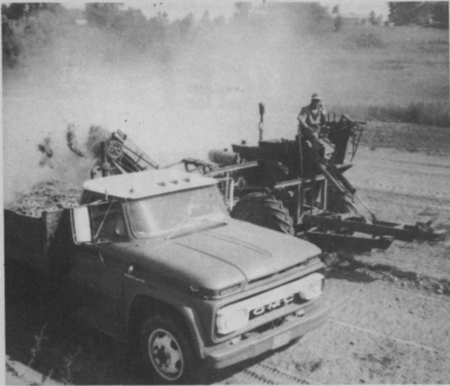
Trucks quickly carry many tons of stones away. Stones are used as the base for greens and future parking areas. The entire operation is highly mechanized.
