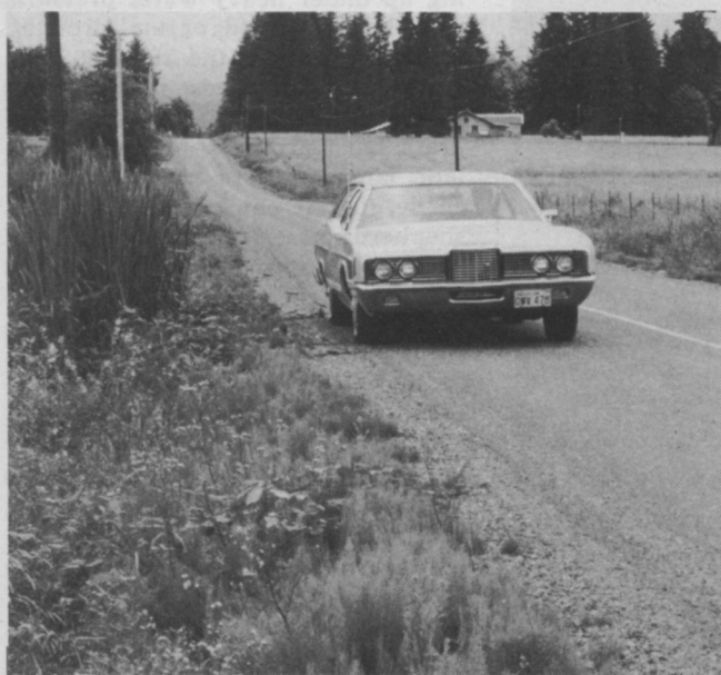
Do you see an 18 inch drainage ditch above? It runs parallel to the road, but weeds and grass have hidden it from view. Vegetation also inhibits orderly water flow and represents a driving hazard.
