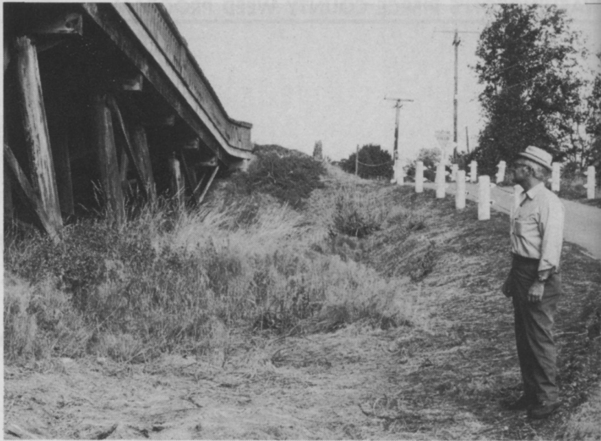
Semi-dormant weeds and grass at base of wooden viaduct shows where weeds and grass have been treated to hold back growth. Without chemical control this growth would be head-high by mid-summer.
