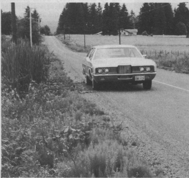
Do you see an 18 inch drainage ditch above? It runs parallel to the road, but weeds and grass have hidden it from view. Vegetation also inhibits orderly water flow and represents a driving hazard.
